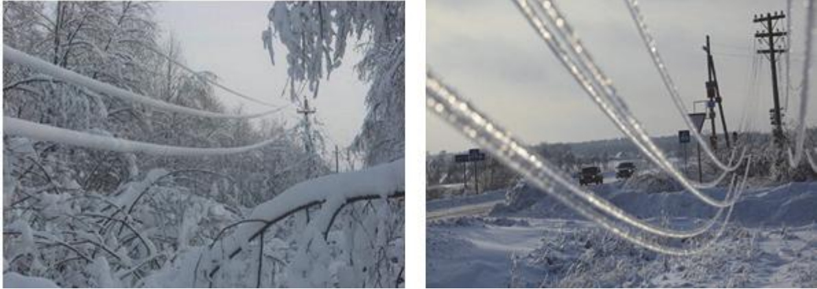
Figure 1. Ice deposits on the wires of overhead power line
