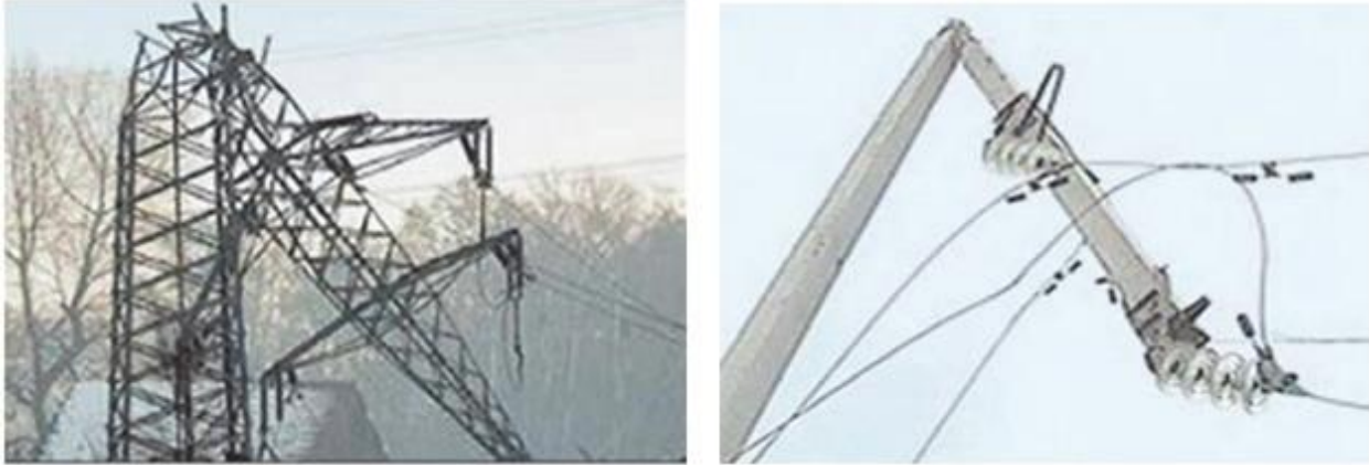
Figure 3. Ice - a disaster for power lines
