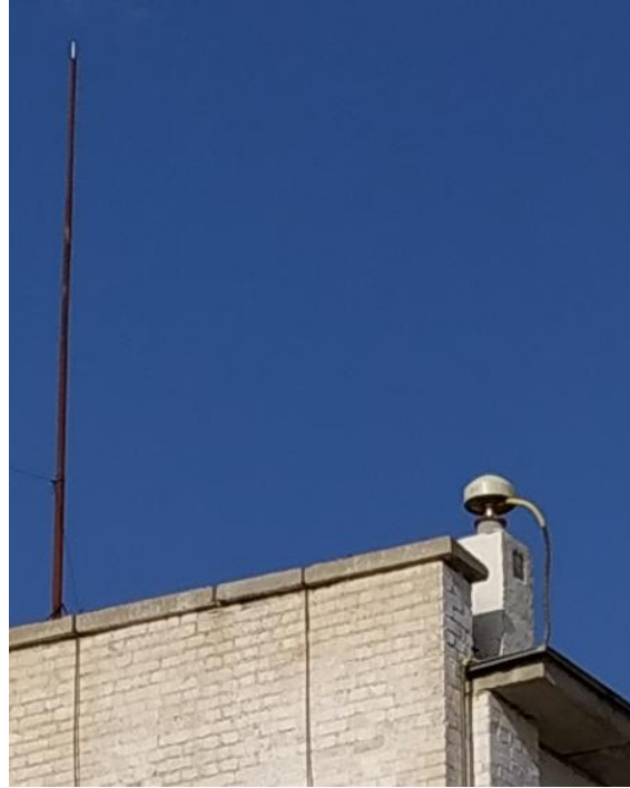
Figure 1. SGS-1 (UCH1) installed in the school building in Uchkuduk.
