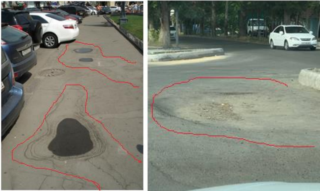
Fig. 3. Dips in the asphalt pavement result from the development of suffusion processes.
