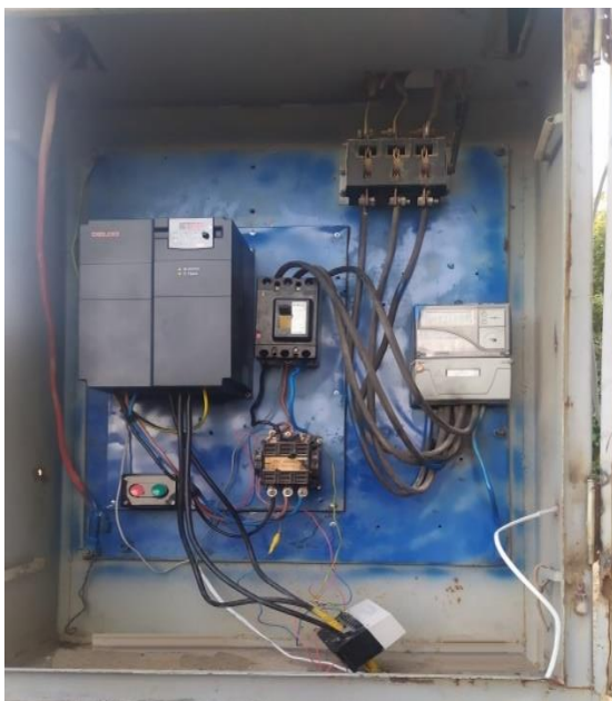
Figure 7. Overview of the installed frequency converter
