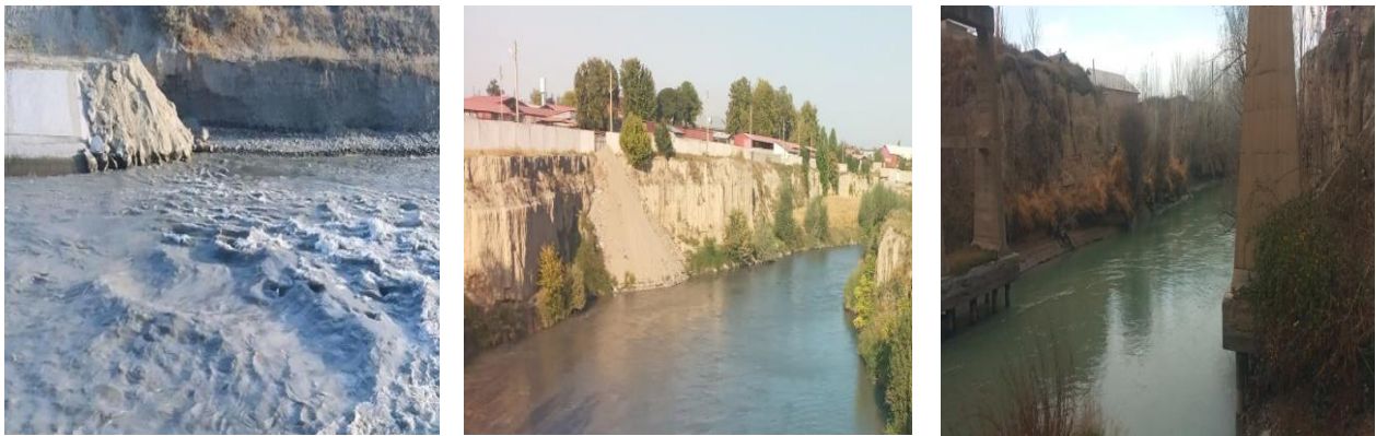
Figure 2. Bank erosion conditions of the Dargom canal
