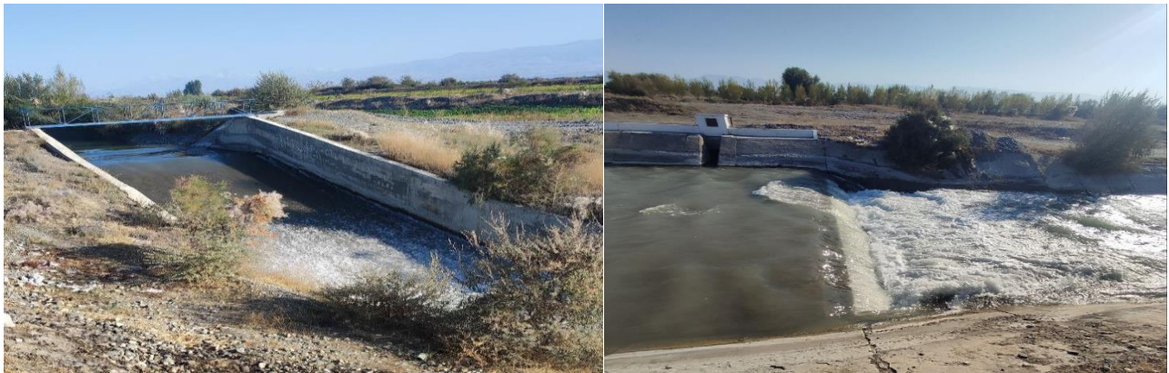
Figure 3. Instances of reducing the kinetic energy of water through the use of rapid flow structures in canal sections PK138+00 to PK153+00
