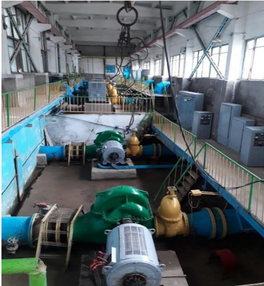
Fig 2. View of the machine Hall of the irrigation pumping station
